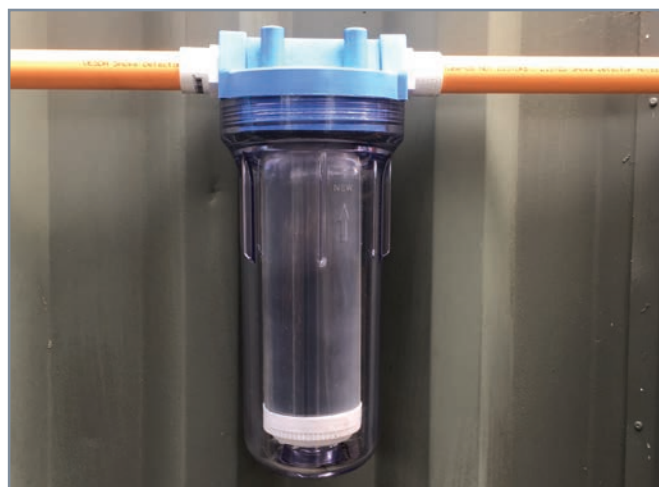
Figure 5 – In Situ Chemical Filters
