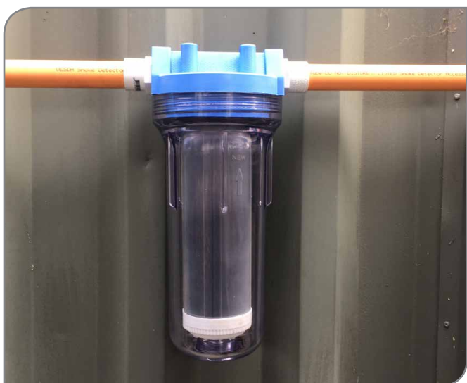
Figure 5 – In Situ Chemical Filters
