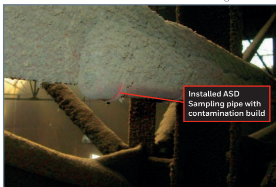
Figure 3: Contaminated sampling pipe
