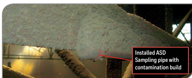
Figure 3 - Contaminated sampling pipe
