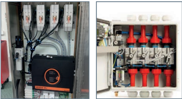
Figure 3: Automated Backflush System
