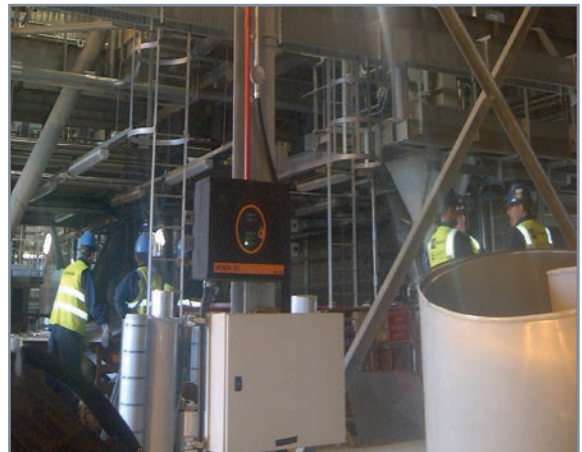
Figure 2 - VESDA detector located in factory where potential EMI exists
