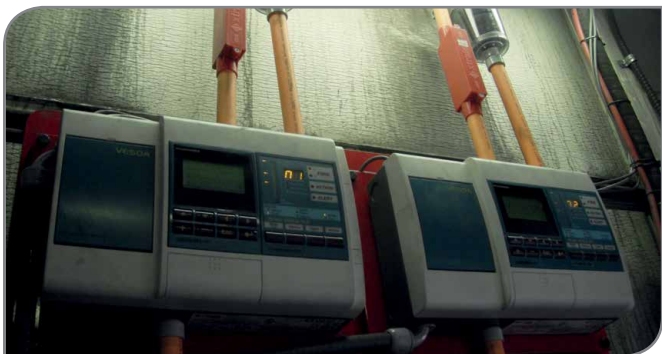
Figure 4 - Detectors mounted in Shovel
