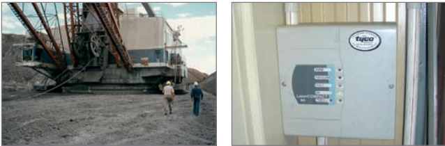
Figure 2 – Dragline with VESDA detector installed
