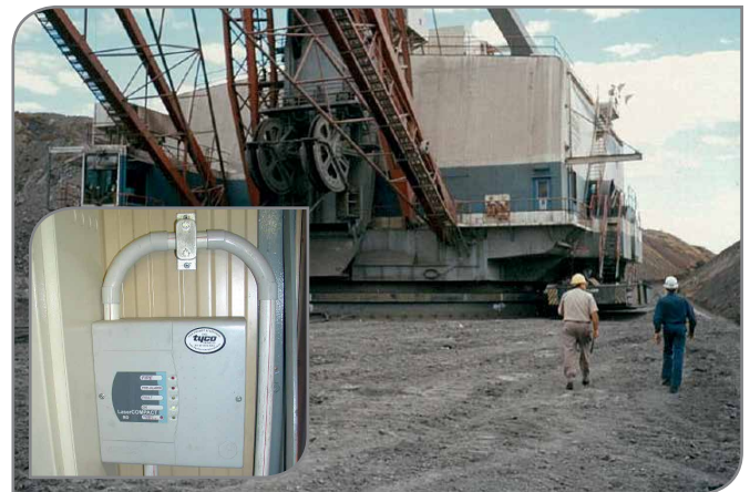
Figure 2 - Dragline with VESDA detector installed
