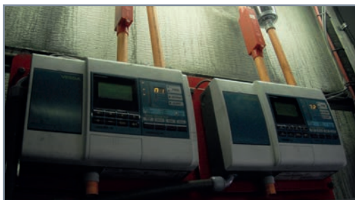
Figure 4 – Detector and Pipes in Roof Space
