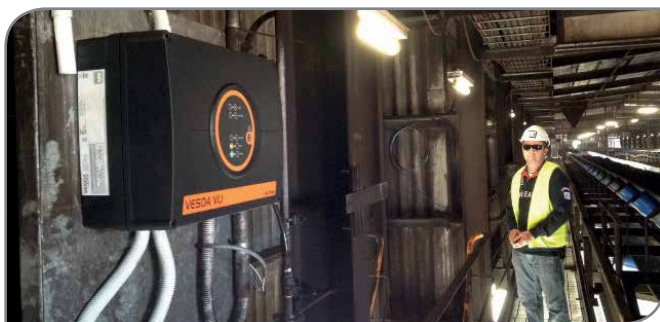
Figure 1 - VESDA VLI in Conveyor tunnel
