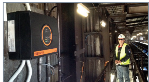
Figure 1 – VESDA VLI in Conveyor tunnel
