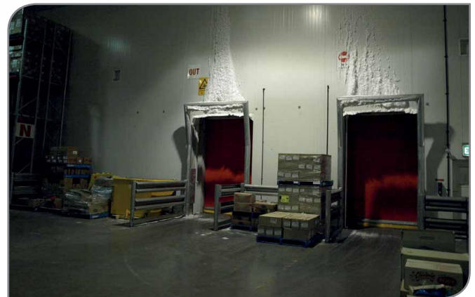
Figure 1 – Icing at entry to cold room
