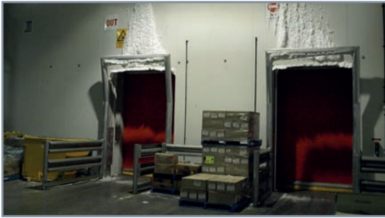
Figure 1 – Icing at entry to cold room
