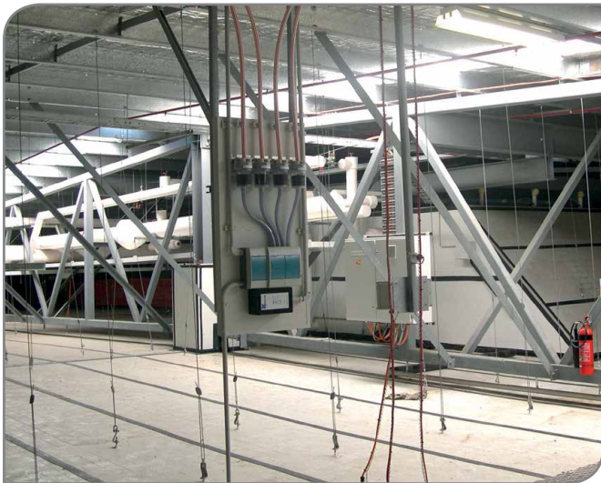
Figure 4 – Detector and Pipes in Roof Space
