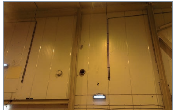
Figure 4 – HFT Sample Pipe within Freezer
