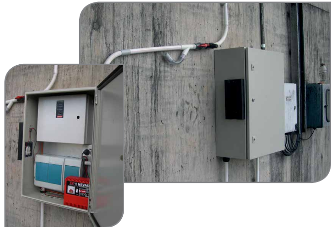
Figure 6 - Thermoelectric Cooling device providing cooling to externally mounted VESDA detector enclosure
