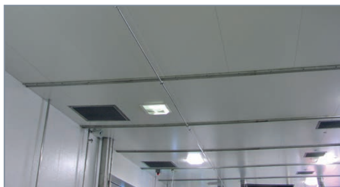
Figure 5: Stainless Steel Sampling Pipe in Poultry Facility
