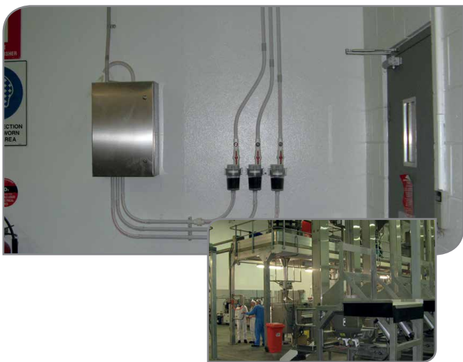
Figure 4 - VESDA System in Food Production Facility
