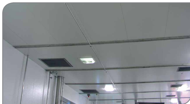
Figure 5 - Stainless Steel Sampling Pipe in Poultry Facility
