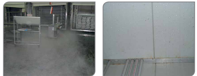
Figure 1 - Condensation on Ceiling Tiles Where VESDA Pipe is Located in Processing Facility
