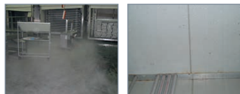
Figure 1: Condensation on Ceiling Tiles Where VESDA Pipe is Located in Processing Facility
