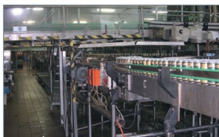
Figure 3: Wet Area Brewery Conveyor
