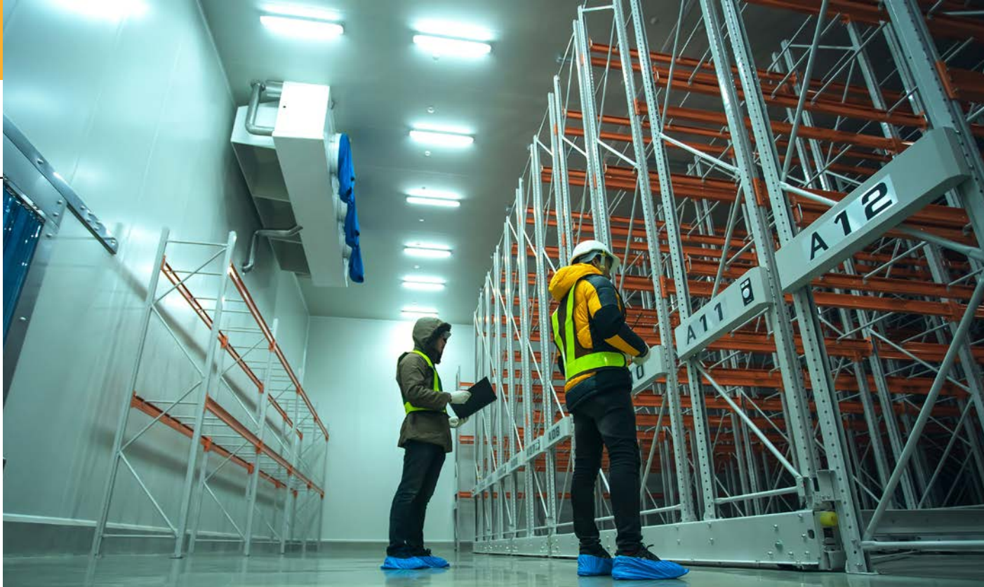
Advanced fire sensing technology detects smoke at the earliest possible stage, while reducing false alarms and maintenance, even in refrigerated and frozen food storage.
