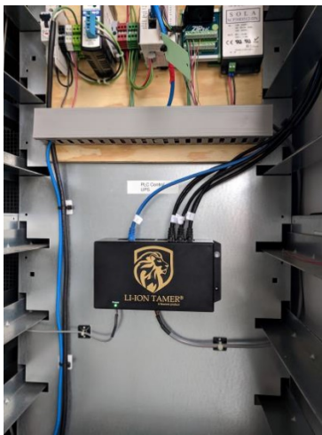
Figure 4: Controllers Tied to System Control Room
