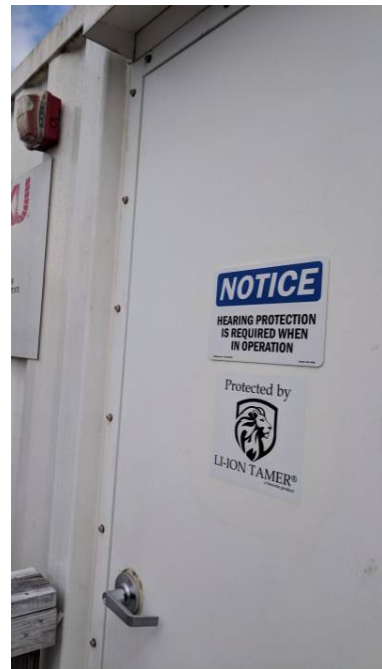
Figure 10: Battery Container Exterior
