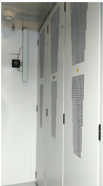
Figure 6: Li-ion Tamer Sensor Placement
