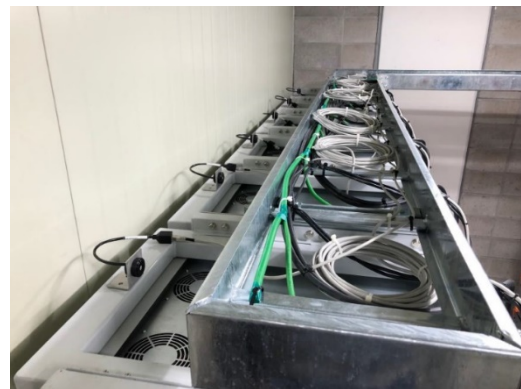
Figure 12: Monitoring Sensors Mounted on Top of Racks
