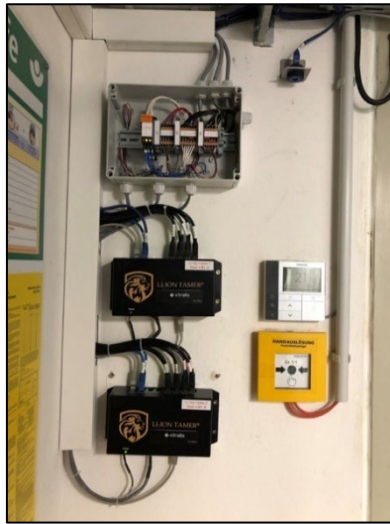
Figure 1: Li-ion Tamer Gen 2+ Controllers
