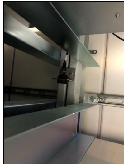
Figure 3: Li-ion Tamer Monitoring Sensor
