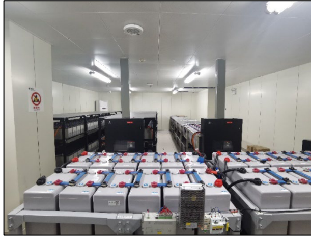
Figure 1: Battery Room (CHIFENG Power Station)
