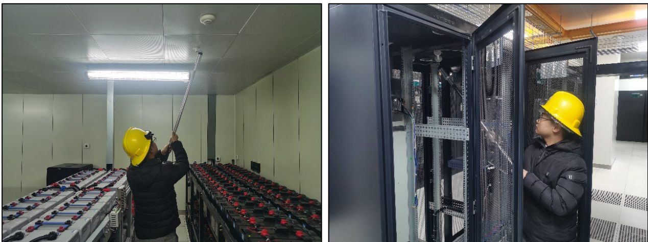
Figure 1: Smoke and Gas Testing in Battery Room
