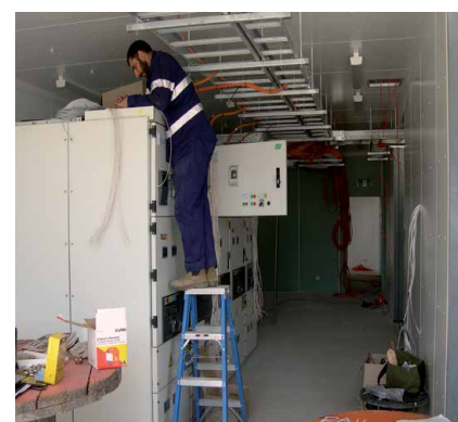
Capillary tubes branch off the main VESDA sampling pipe and into the equipment cabinet, allowing the earliest possible warning of smoke within the cabinet.
