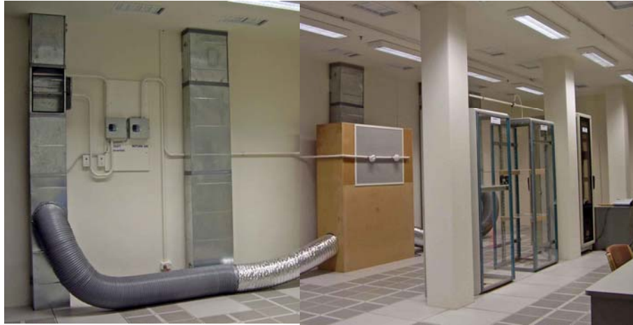
Figure 1 – Xtralis Test Facility IT/server Room.
