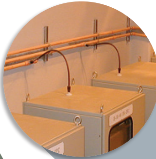
Capillary tubes sampling inside cabinets provide reliable equipment protection.
