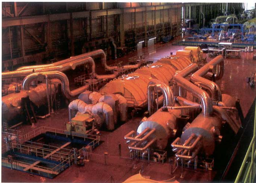
A massive turbine at Bruce Power’s plant in Ontario, Canada.
