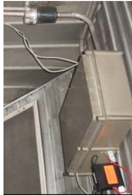
Figure 3 ECO Installation – VESDA Exhaust
