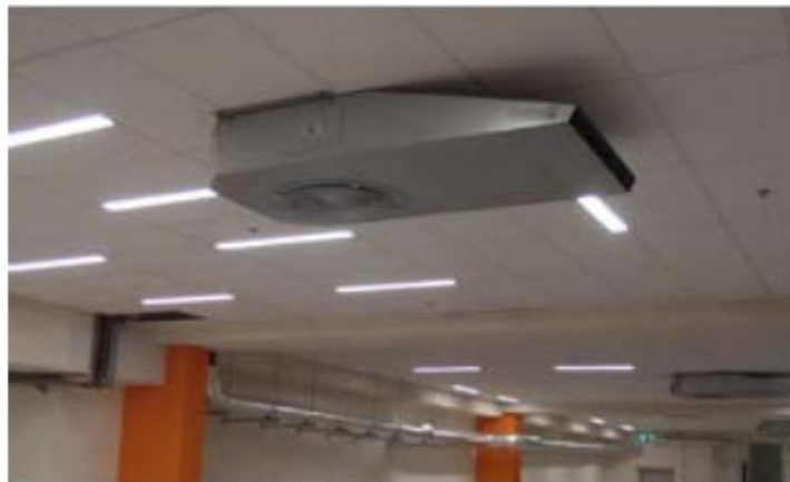
Figure 1: Impulse Ventilation Fan in Car Park (cyclone induction type)
